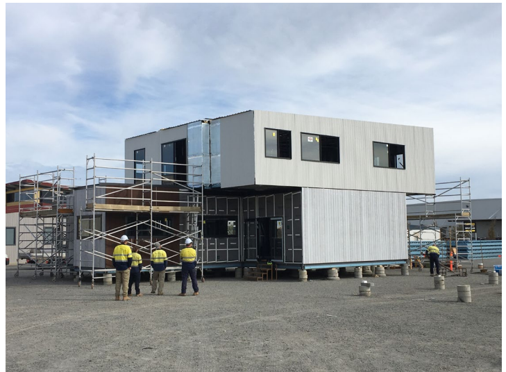
Figure 4 Legacy Living Lab during assembly at Fleetwood, June 2019. The Lab will be in place at East Village, Fremantle, in August/September 2019
