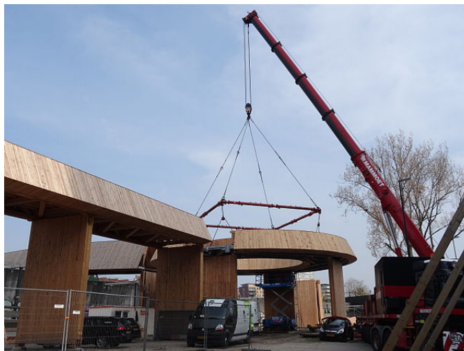
Luchtsingel bridge under construction. Photo by AgainErick via Wikimedia Commons CC BY-SA 3.0
