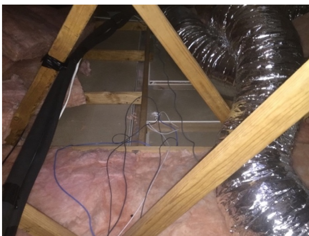
Figure 19. Missing ceiling insulation in roof space (Source: Munsami 2018)
