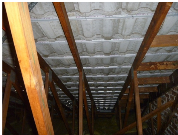
Figure 16. Gaps between tiles are clearly visible in an unsarked roof (Source: Munsami 2018)
