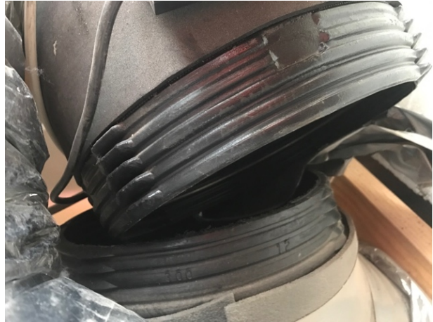
Figure 29. Disjointed duct in the attic of a house in Sydney (Source: Munsami 2018)
