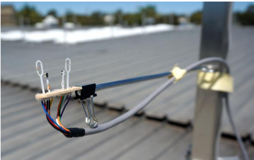
Figure 3.4: Wind measurement assembly, consisting of two horizontally opposed sensors, installed on a 1.5m mast.
