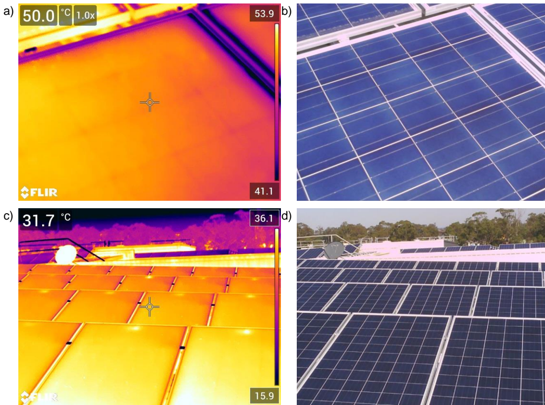
Figure 3.13: Comparison of thermal and visible images of PV panels, taken in Shellharbour (a and b) and Wetherill Park (c and d).
