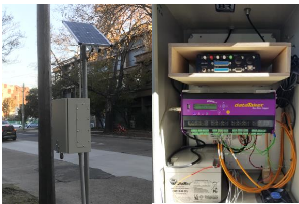
Figure 14. Solar powered data logger installation.
