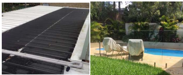
Figure 1 Residential solar pool heating system.
