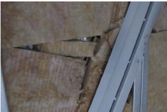
Figure 24 - Poor installation of the insulation
