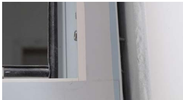
Figure 21 - Window frame and waterproofing detailing problem
