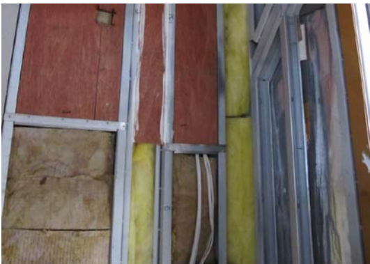
Figure 25 - Mix of insulation types used and no thermal breaks in a structure that it is mostly steel
