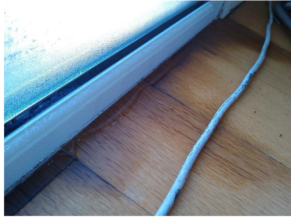
Figure 18 - Condensation in the frame and glass on the south window of bedroom 3
