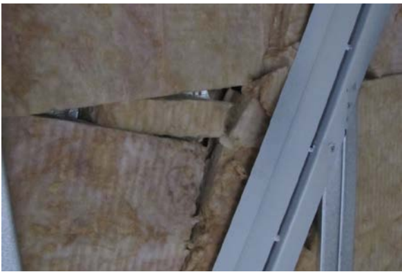
Figure 24 - Poor installation of the insulation
