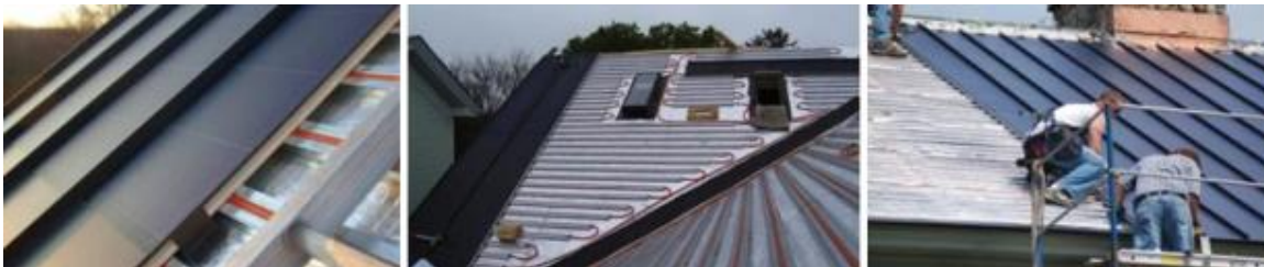
Figure 28: Dawn Solar SunNet BIPV using UniSolar P/Thermal system on an Englert metal roof
