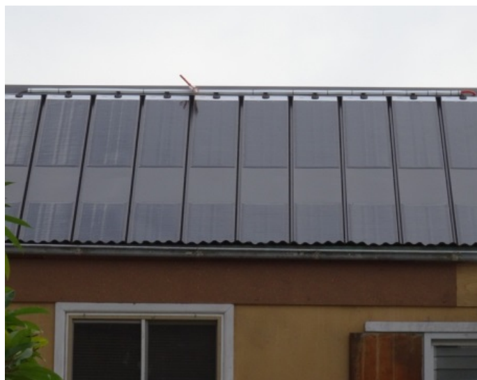
Figure 1- Bluescope BIPVT on a House in Sydney
