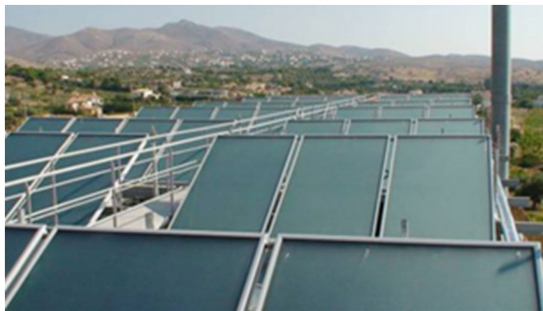
Solar thermal collectors on top of an office building in Greece.
