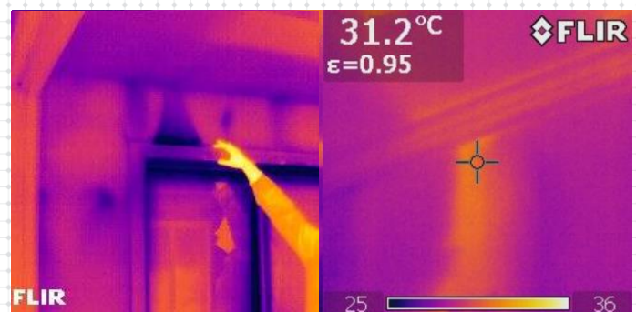
Fig. Thermal imaging shows air infiltration
