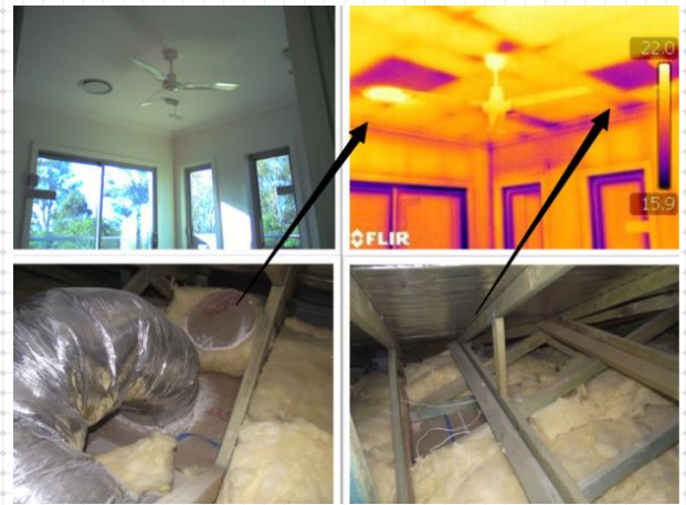
Fig. Our thermal camera proved effective at identifying insulation imperfection and led us to discover that two insulation batts were missing.
