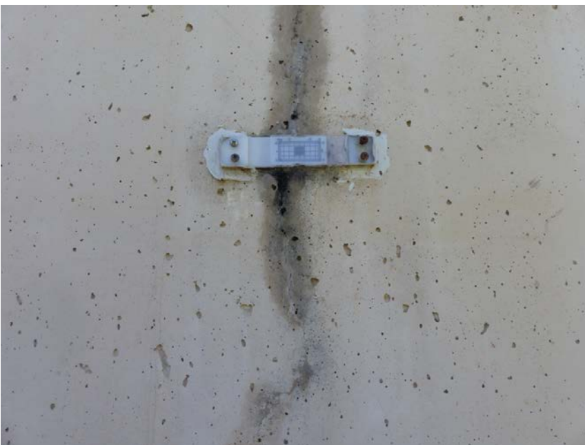
Figure 14. Surface crack of Geopolymer concrete water tank at Toowoomba site, QLD, in December 2015.
