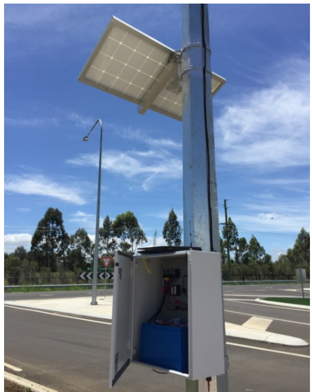
Figure 75. Solar power supply system used at Toowoomba Bridge site, QLD.
