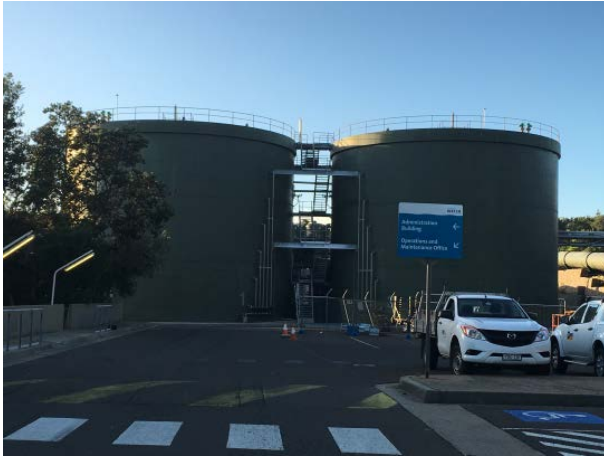
(a) Digesters 1 (left) and 3 (right).
