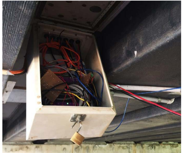
Figure 74. Control box of the monitoring system at Toowoomba Bridge site, QLD.
