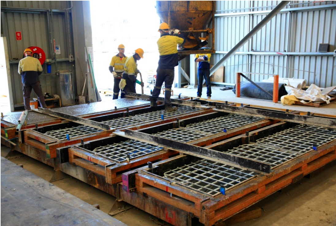
Figure 101. Concrete casting of four boat ramp planks at Wagners precast yard at Wacol, Queensland.
