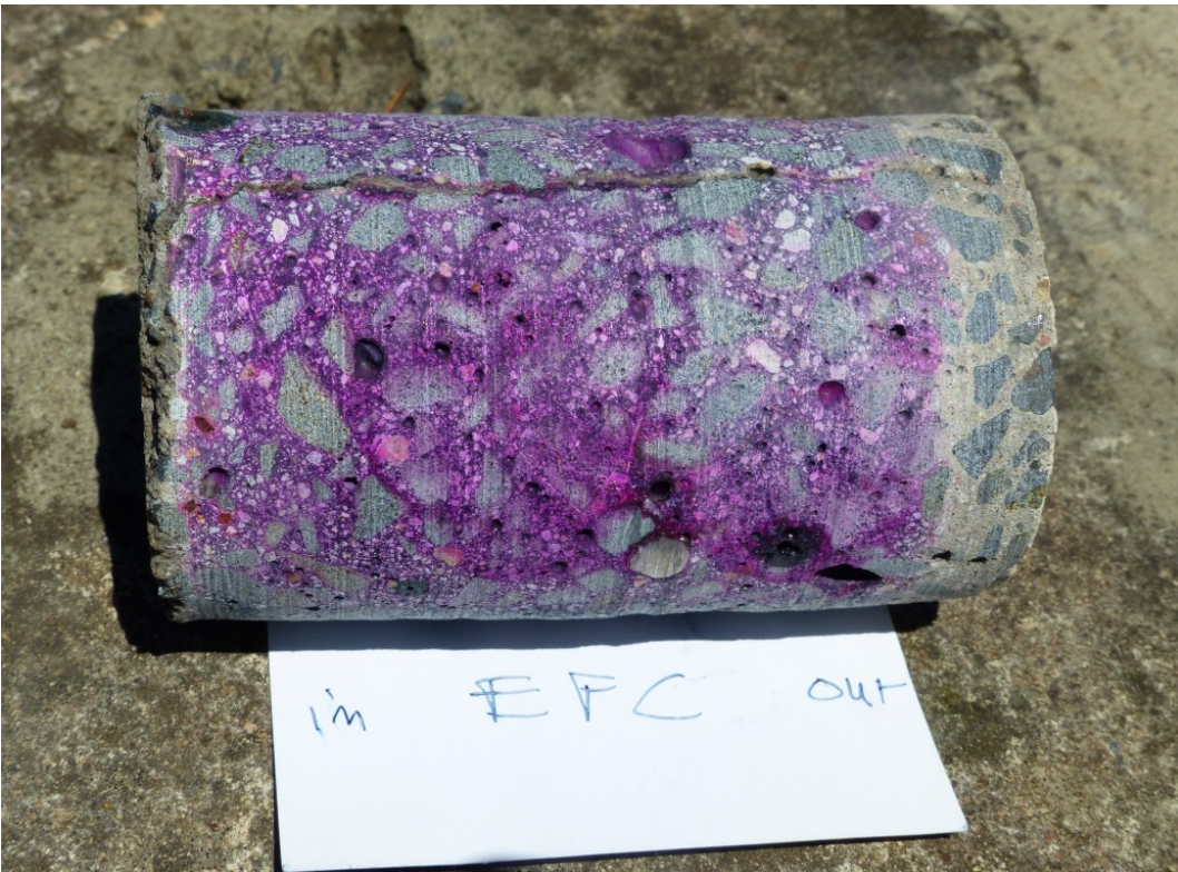
Figure 16. Geopolymer concrete core taken from water tanks at Toowoomba Site, QLD, in December 2015.
