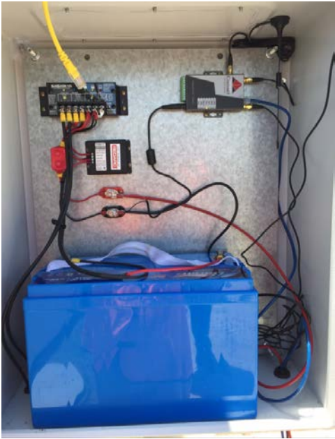
Figure 76. Interior view of the solar control box at Toowoomba Bridge site, QLD.
