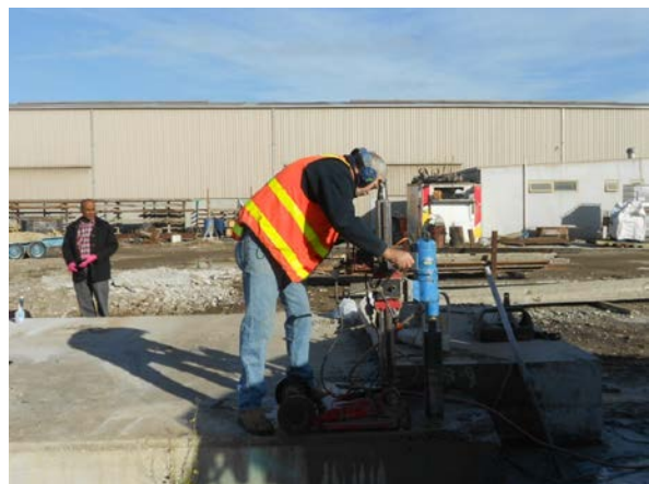
Figure 3. Extraction of cores from main slab at Campbellfield site, VIC in April 2015.
