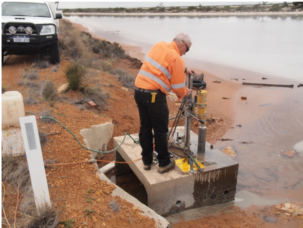
Figure 23. Coring of Geopolymer concrete culvert at Lake King site, WA, in October 2015.
