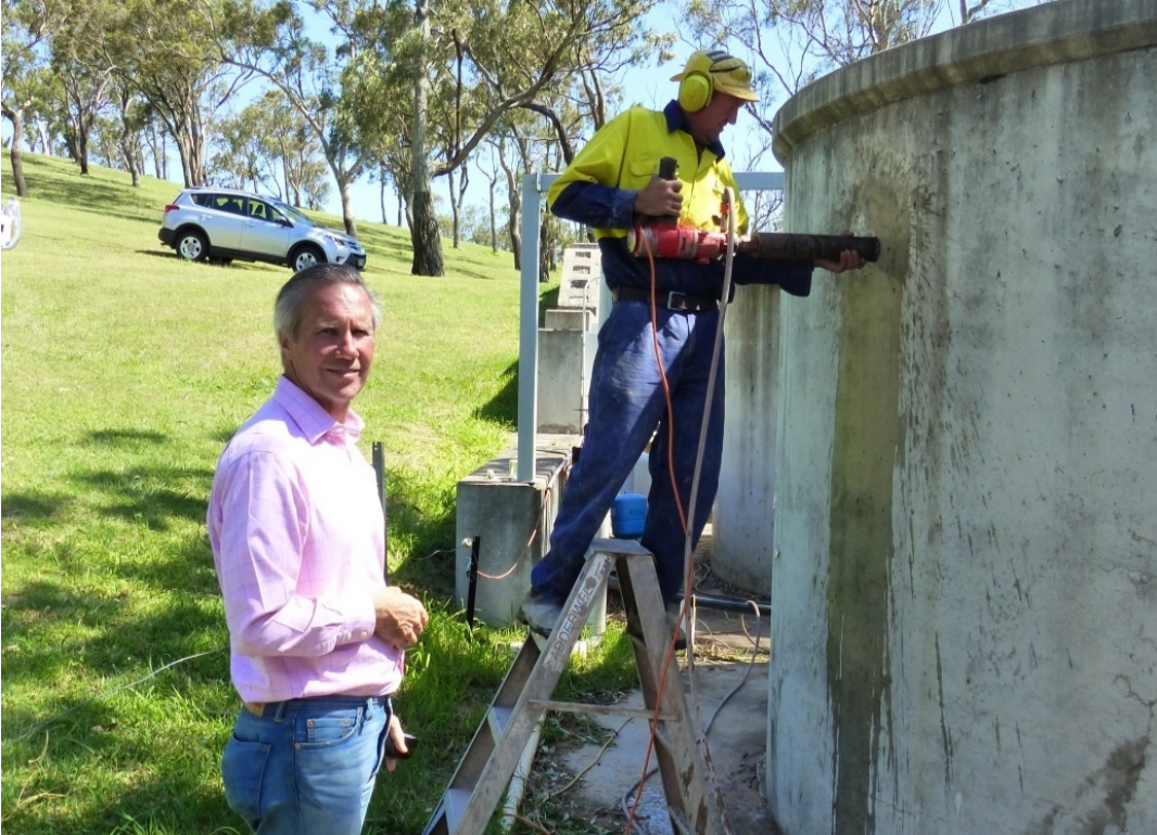
Figure 15. Coring of OPC concrete water tank at Toowoomba site, QLD, in December 2015.
