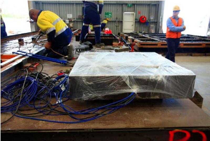
Figure 112. Precast EFC panel with sensors embedded at Wacol, QLD, and ready for transport to site (June 2016).
