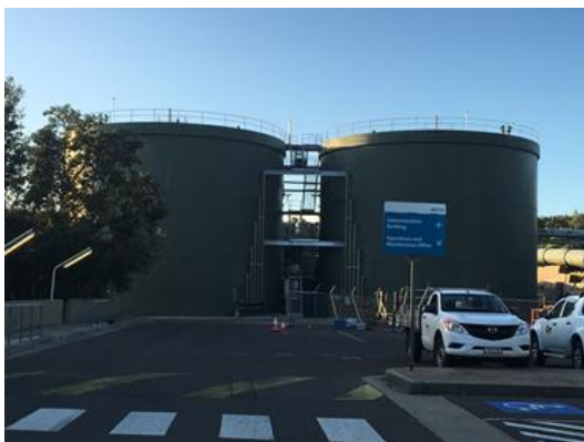
(a) Digester 1 (left) and 3 (right).
