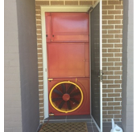
Figure 15: Blower door tests for BASIX-compliant dwellings with high space heating and cooling energy consumption (Munsami, 2019)
