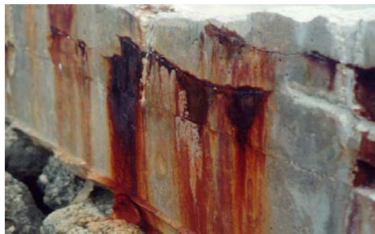
Figure 1: Corrosion of reinforcing bars leads to serious problems with millions of dollars spent for maintenance, repair or replacement of damaged structures.
