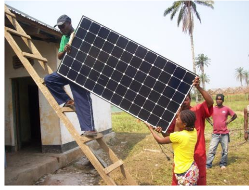
Figure 16. Village solar installation. © Greenpeace
