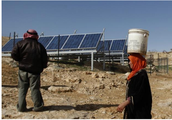
Figure 15. Solar installation in Gaza. © Jersualem Post
